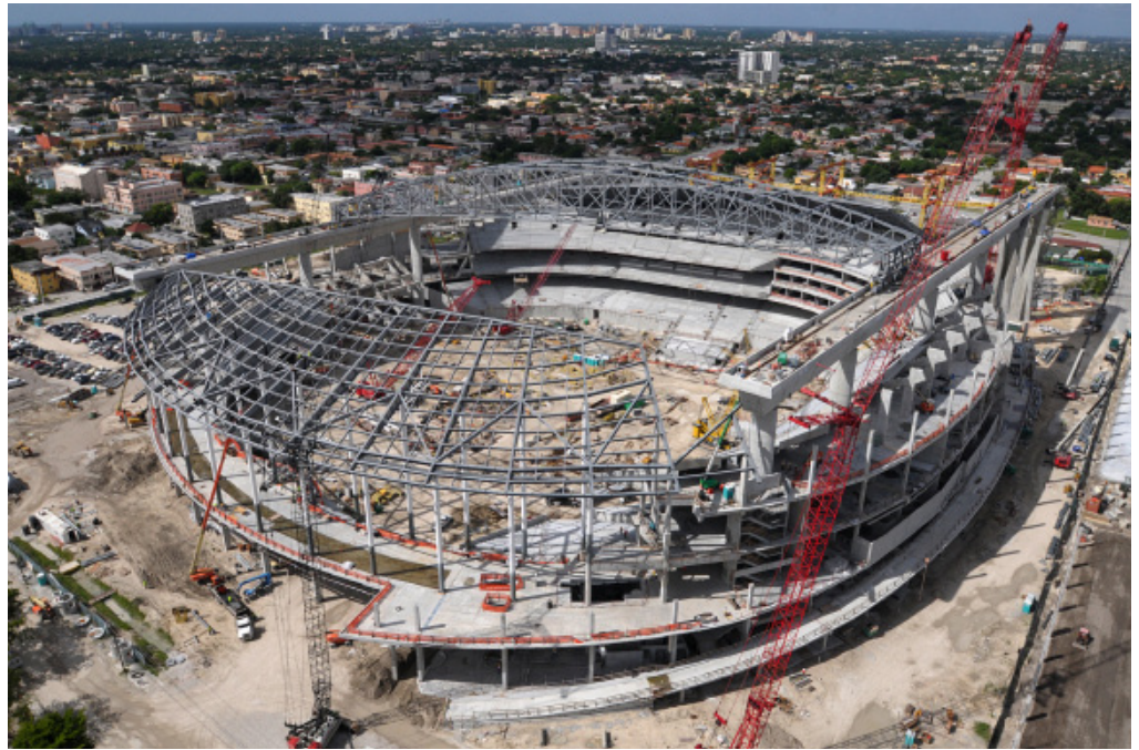
Aerial photograph of the ballpark under construction. Image courtesy of Hunt/Moss. Photo by Aerial Photography, Inc.
