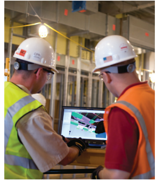
Autodesk Navisworks model being used at the construction site. Image courtesy of Robins & Morton.
